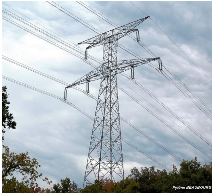
Figure 2-6 Example of a 440 kV Double-Circuit Transmission Line
